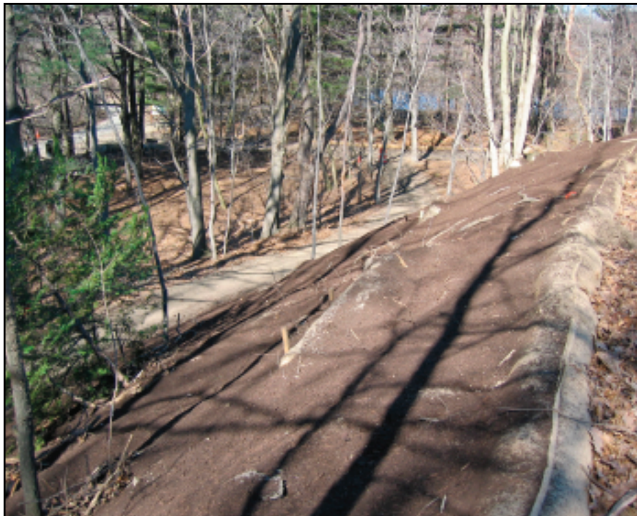
More than 206,000 square feet of EarthBlanket™ were installed hydraulically to provide erosion management for steep slopes surrounding Fresh Pond Reservoir. Photo credit: Thomas Benjamin, VHB, Inc.
