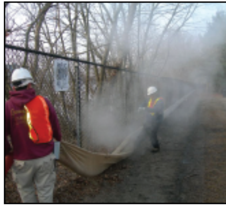
Installation of FilterMitts was key in the protection of public drinking water. Photo credit: Phase II Stormwater Products.
