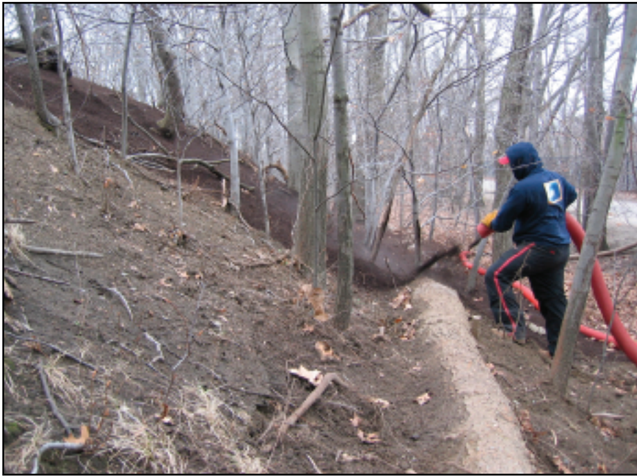
Installation of the proprietary compost blanket product that was chosen because it not only stabilizes the slopes, but also cleans the water. Photo credit: Thomas Benjamin, VHB, Inc.
